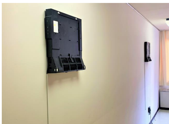
Photo 1: Photocatalyst sterilizer/deodorizer installed on the wall of the hospital room
